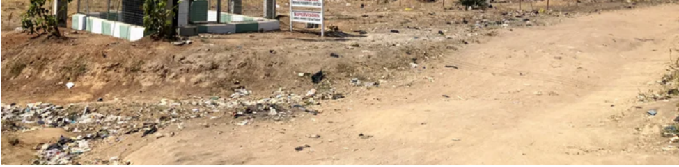
Nigeria's power grid—including infrastructure like this 33/0.415 kilovolt substation in a community near Abuja Airport—fails to reach a significant percentage of the population. LUCAS LAURSEN
